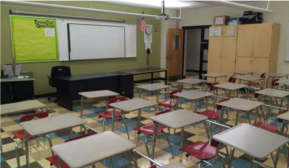
2,241 LED Direct/ Indirect Retrofit
